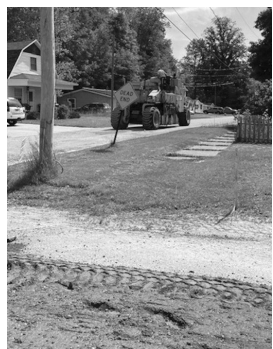
Starting June 8, nine streets in Boyer City will receive $275,005 of capital preventative maintenance repairs. Courtesy photo
